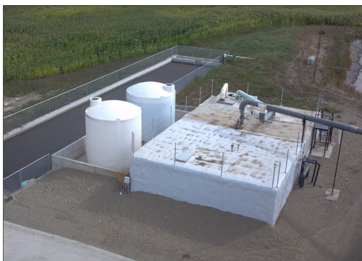
Figure 2. Commercial-scale phosphorus and nitrogen nutrient recovery facility integrated with a dairy anaerobic digester, Lynden, WA. Photo courtesy of Eric Powell.
