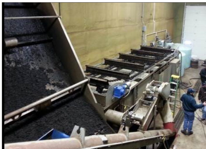
Figure 3. Commercial-scale recovery of phosphorus solids, integrated with a dairy anaerobic digester in Bio-Town, IN. Photo courtesy of Doug Van Ornum.
